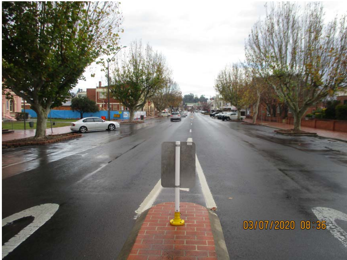
Photo 9 – Otho Street road formation (viewed from pedestrian crossing between Council Chambers and Government Offices)
